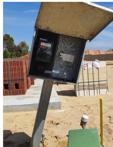
Support structure unstable
