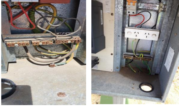
Compromised IP rating
